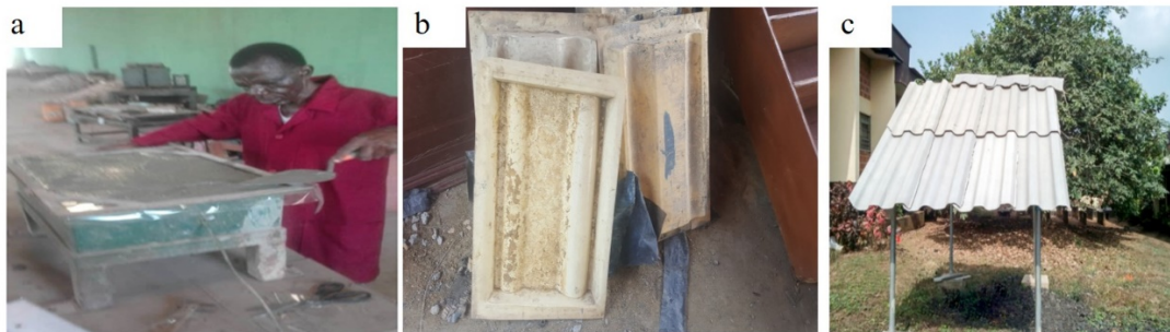
Fig 5: (a) Placing the mix on the Vibrating Machine (b) Mador Tiles as Produced (c) Application of the Mador Tiles
