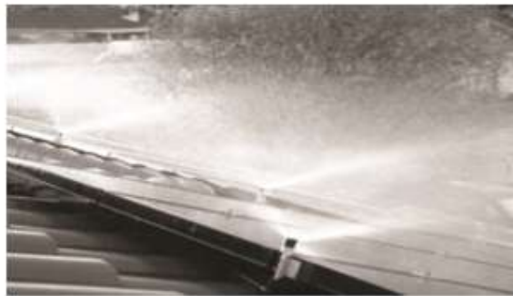
Fig. 2. Fully automated water cleaning system Source: (H. A. Kazem et al., 2020)
